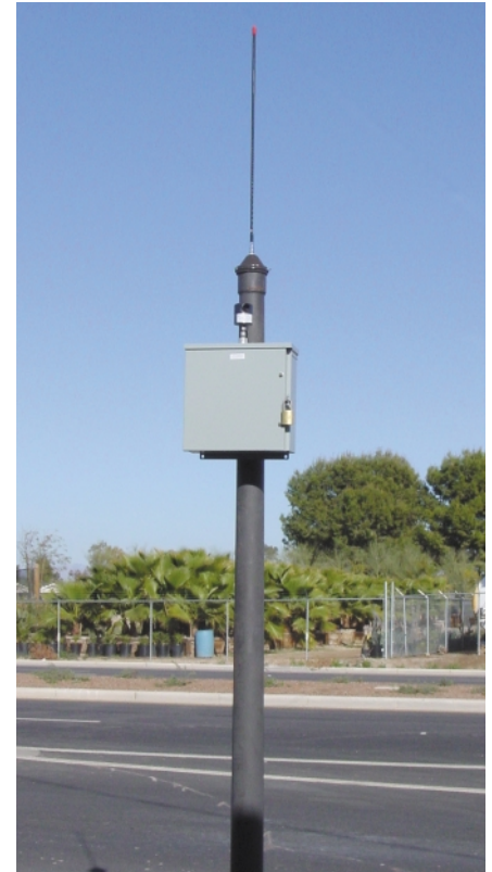
Optical sensor with radio transmitter at end of fire station driveway.
