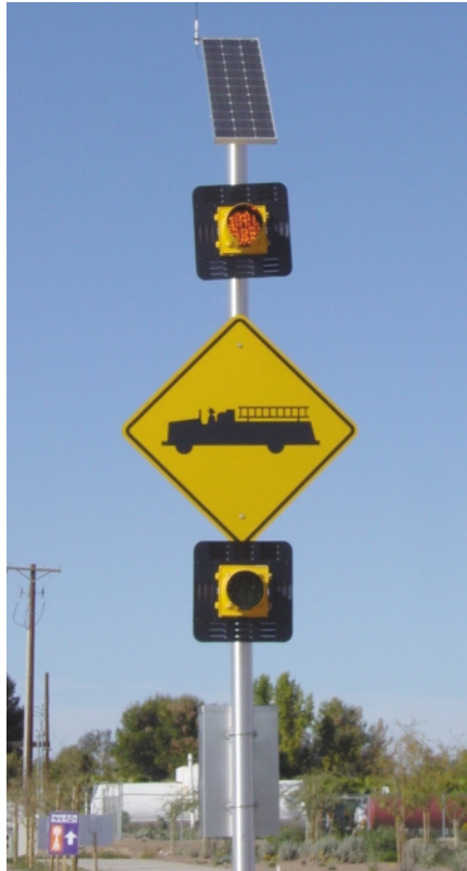
Typical Type I radio-activated fire station flasher.
