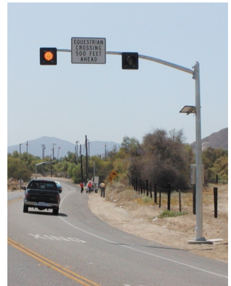
Mast-arm flasher slows down approaching vehicles.
