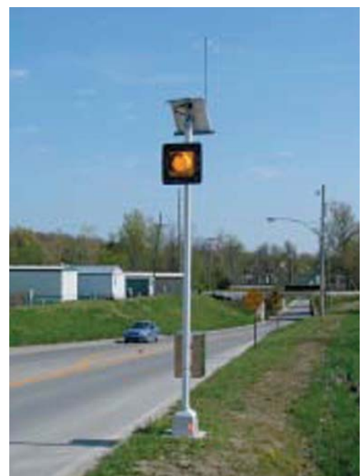
Southbound flashing beacon assembly
