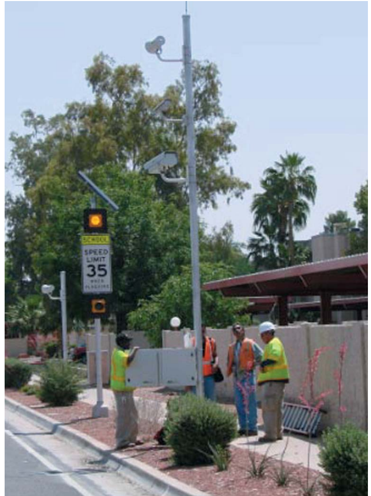
Personnel from American Traffic Solutions and STC install the photo radar interface to existing flasher system.
