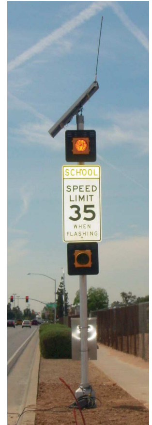
City of Mesa school zone flasher along Baseline Road
