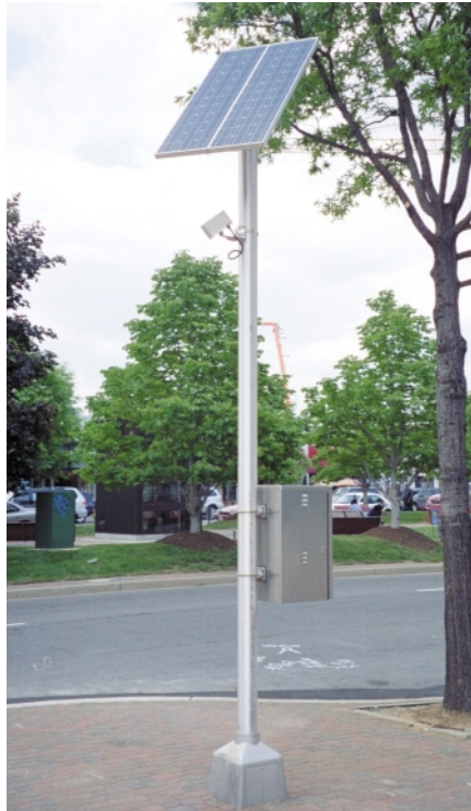
Sensor station for sensor-activated crosswalk flasher. Photo courtesy of Randy Dominick, Traffic Systems & Technology.
