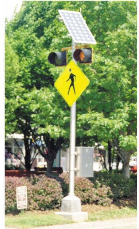
Dual 12-inch, flashing beacon system upstream from the crosswalk. Photo courtesy of Randy Dominick, Traffic Systems & Technology.
