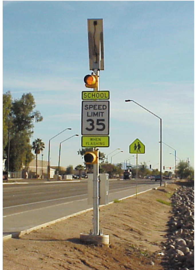
Solar panel faces south for optimum exposure to the sun.
